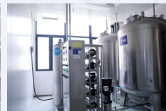
Water Treatment Room
